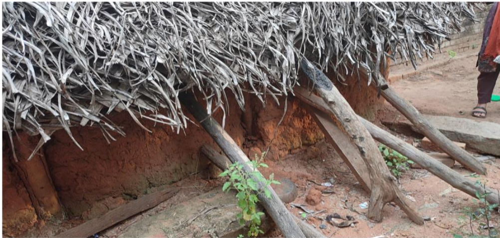
Most of the CIHs had walls and roofs that were weak and vulnerable to heavy rains and cyclones.
